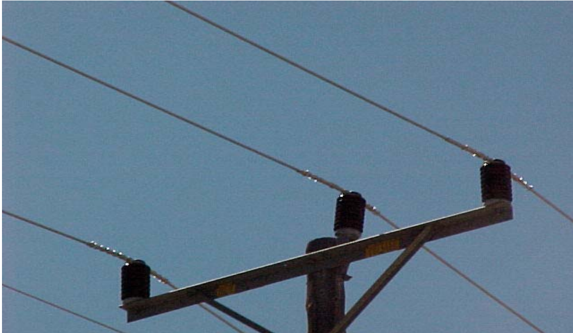
Portal Powerhouse Grid Interconnect sub-transmission line without raptor hoods.
