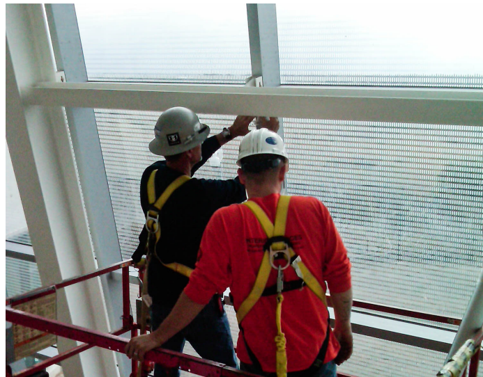
Workers are installing mechanical window shades that are operated by a control system to optimize energy efficiency and lighting level throughout the day.
