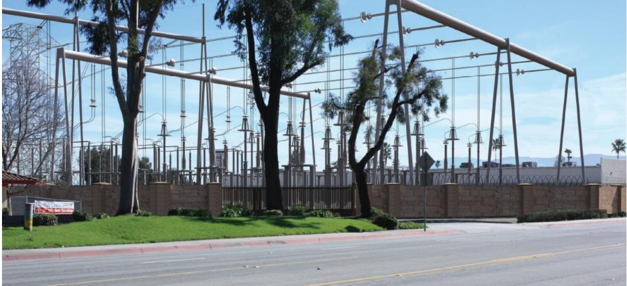
Simulated view looking southeast from Pipeline Avenue toward the proposed Eastern Transition Station in Chino Hills as part of TRTP 500 kV Underground.
