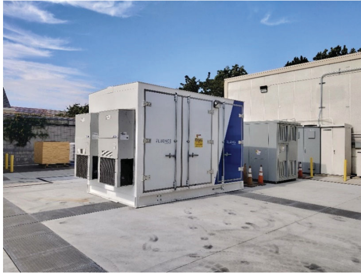
Figure 2. Fully Installed DPC
