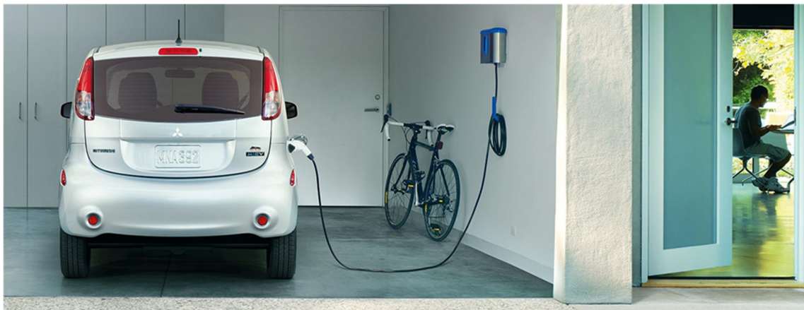
Figure 2. Residential EV Charging Example
