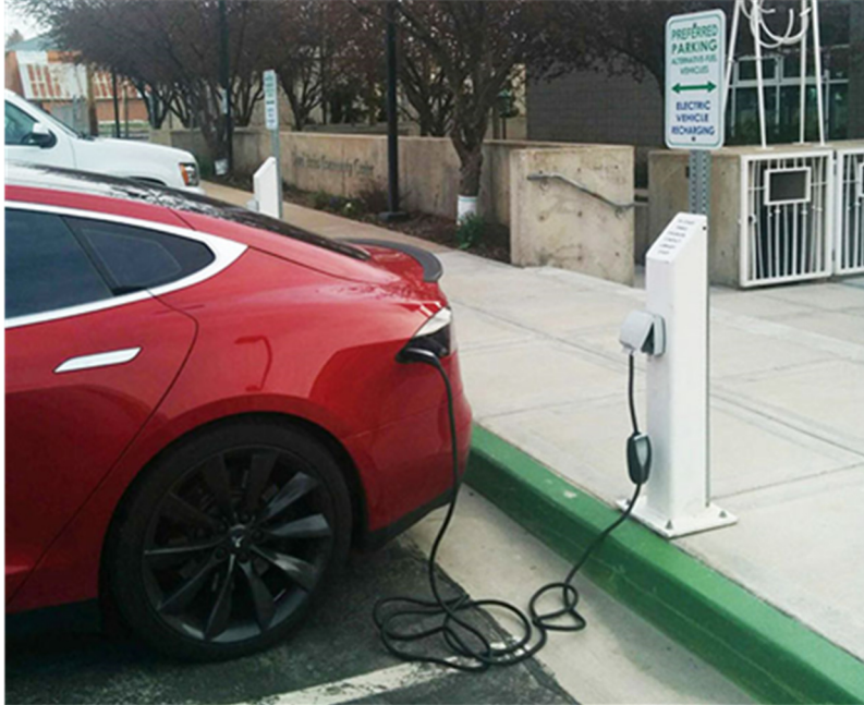
Figure 3. Commercial EV Charging Example
