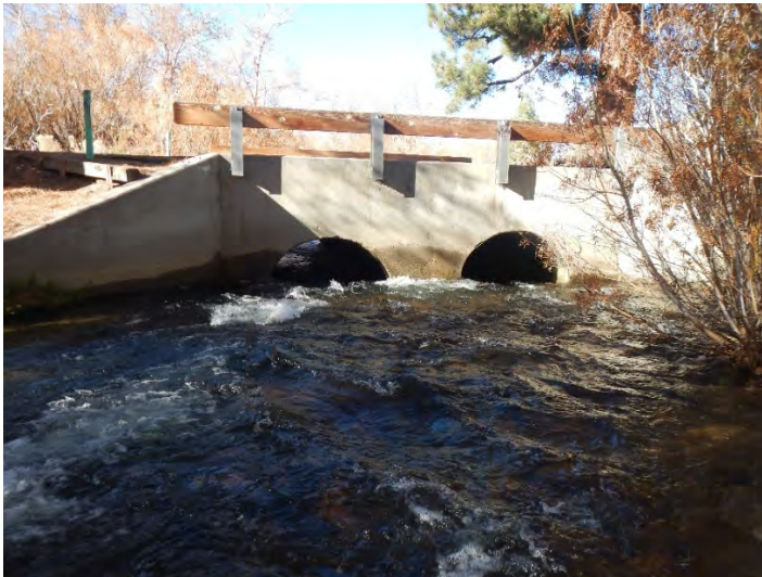
PHOTO C- 17 TRANSECT 9-2 AT LOW FLOW, 8 CFS (LEFT), MID-FLOW, 20 CFS (RIGHT), AND HIGH FLOW, 40 CFS (BOTTOM), CONDITIONS. ORIENTED DOWNSTREAM.
