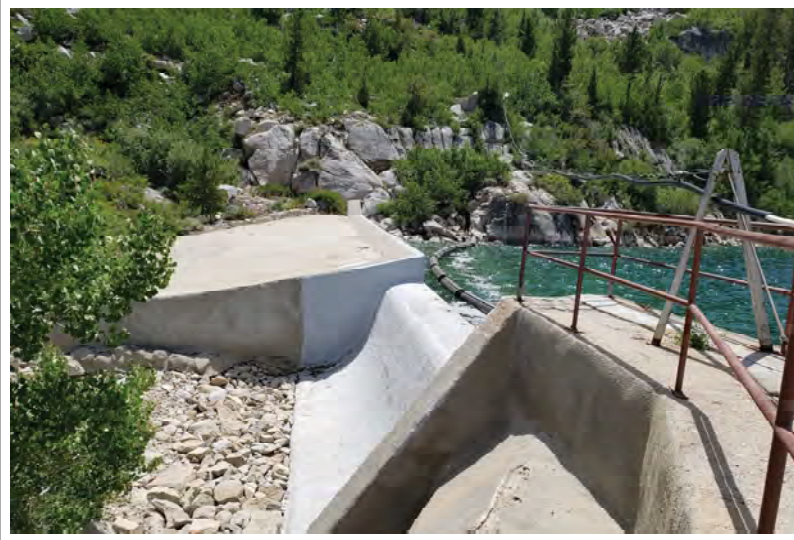
Photo 9: View of the diversion dam and surrounding habitat at the Birch Creek Diversion.
