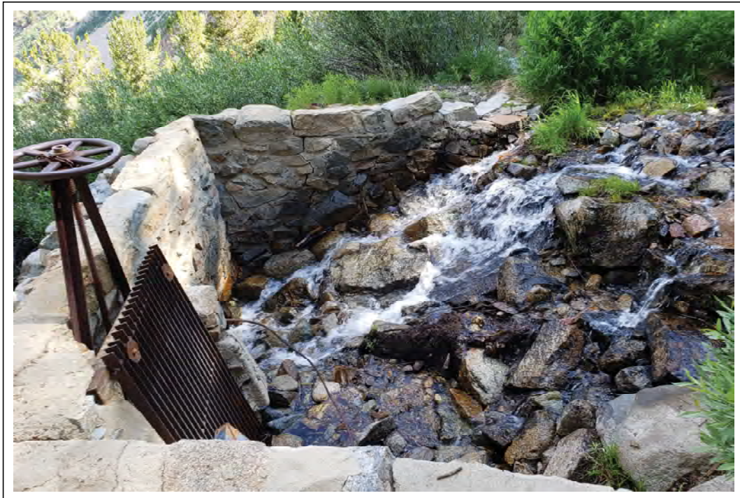
Photo 8: View of the diversion dam and surrounding habitat at the Green Creek Diversion.
