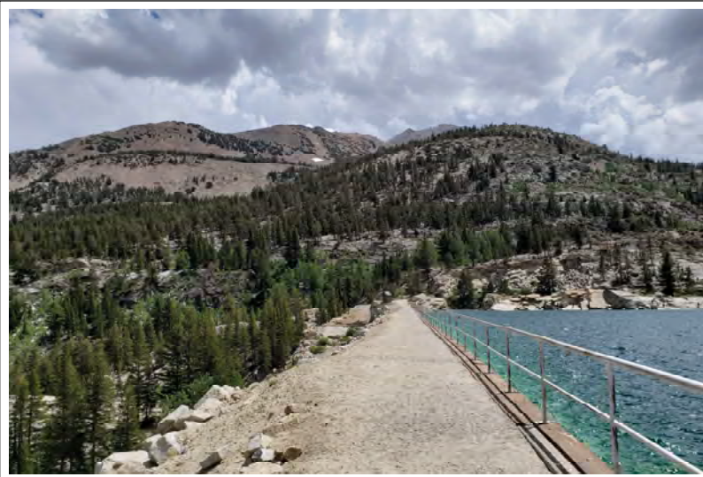
Photo 10: View of the diversion dam and surrounding habitat at the McGee Creek Diversion.
