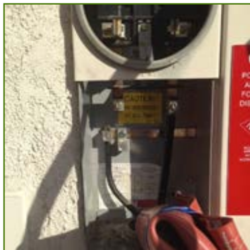
Exhibit #2 Completed Meter + GMA installation + wiring
