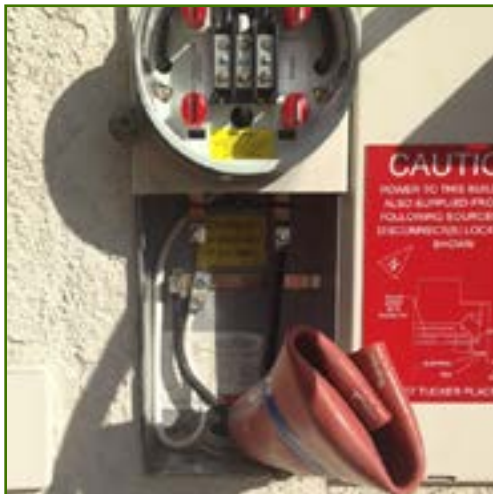
Exhibit #2 GMA installation
