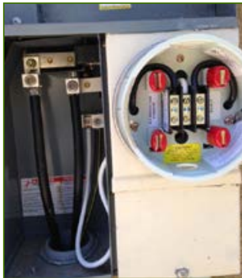
Exhibit #1: Multi-port connection
