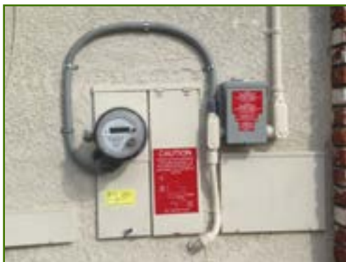
Exhibit #2 Completed Meter
