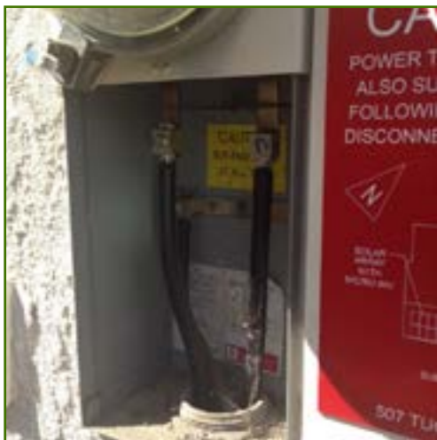
Exhibit #1 Panel Wiring
