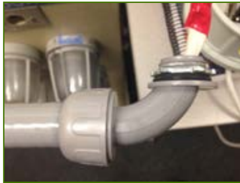
Red tape around section of pump/ Bent Connector
