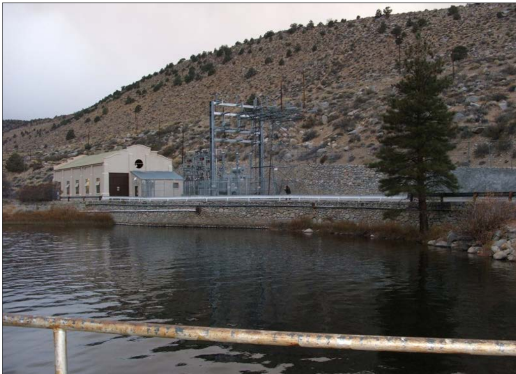
Photo 9.10-8. Plant No. 3/Intake No. 4 Facilities
