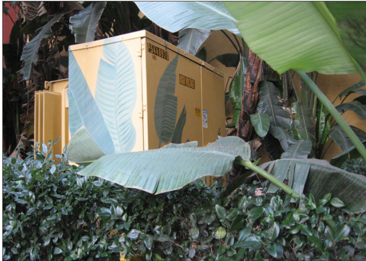
SCE offers several options to lessen the visual impact of above-ground distribution pad-mount equipment, including painting and installing digital wrap films. (Note: Customers must maintain adequate clearances and access to SCE equipment.)
