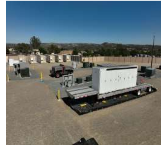
MBESS at Cameron Corners Microgrid
